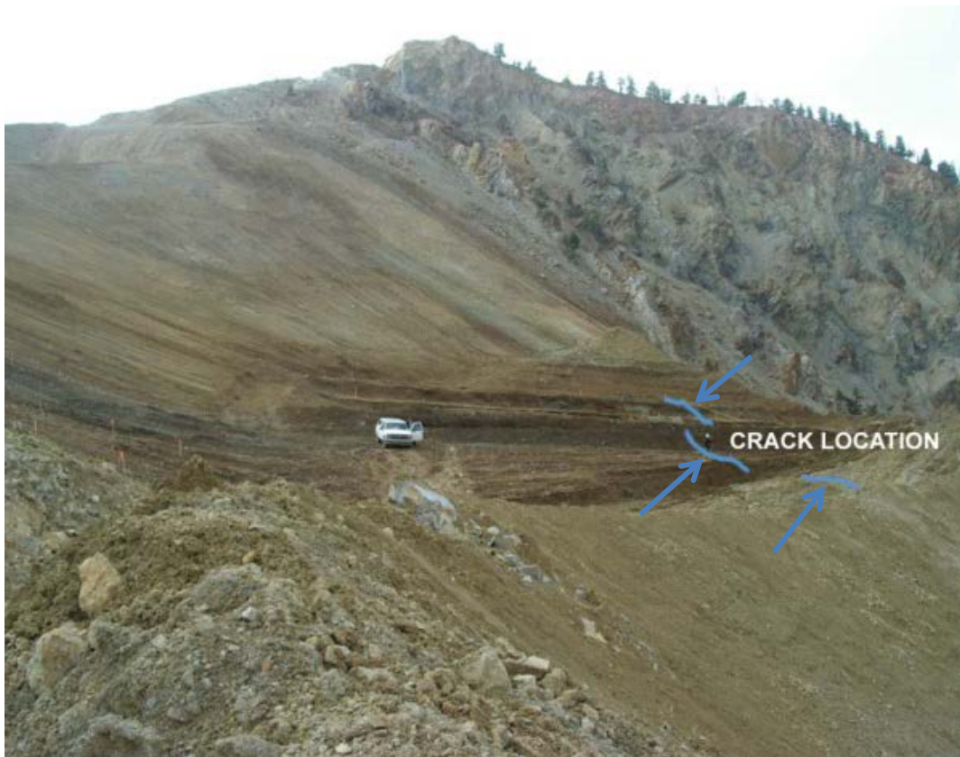
Figure 3 Approximate crack locations from the side of the slope (highlighted in blue)
